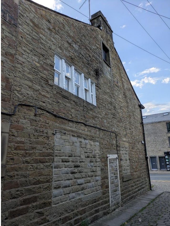
The return of the Duke of Buccleugh, a possibly earlier, re-fronted building with evidence of weaving windows and a taking-in door (now blocked to form window) in the attic space.
