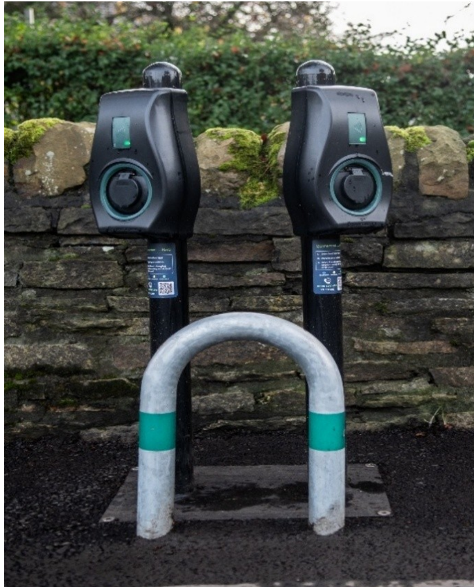
Figure 7-Connected Kerb On-Street Residential EV Charging Infrastructure in Rossendale
