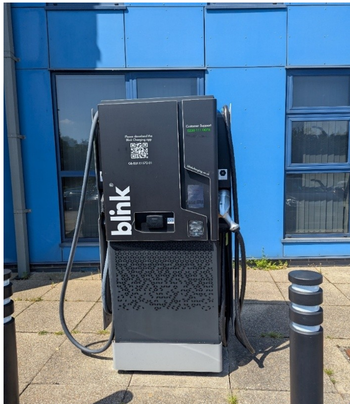
Figure 8- Blink Rapid AC/DC EV Charge Point at Futures Park, Rossendale
