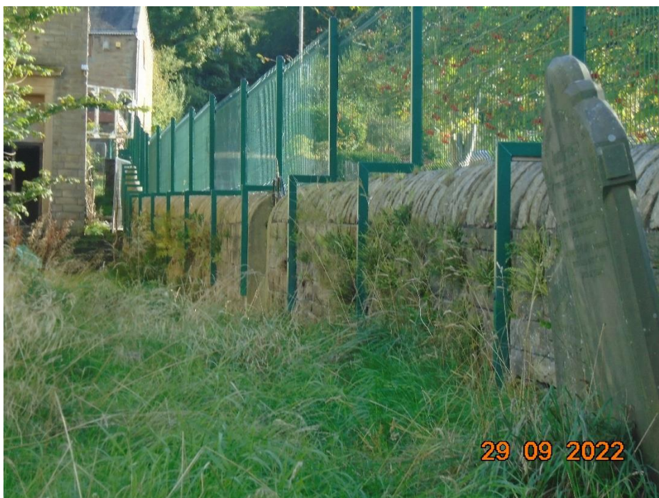
View from the graveyard behind the Rakehead Lane Wall. Courtesy of Enforcement Officer.
